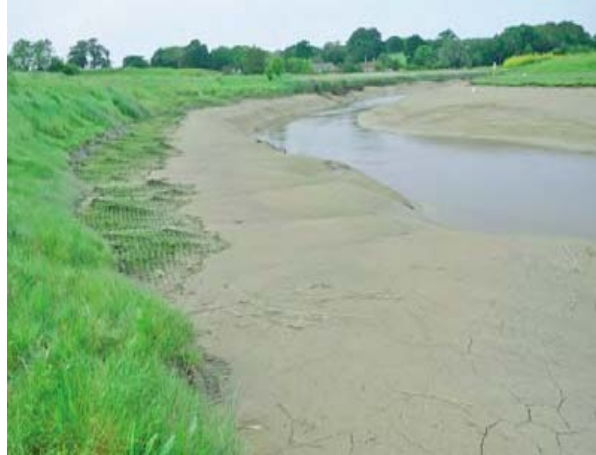
Seven years post-restoration the structure has continued to retain sediments and has been stabilised further by vegetation
