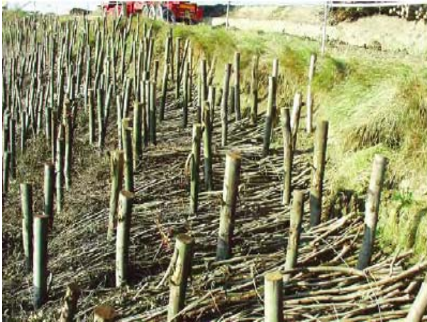
Once brushwood mattress installation is complete, rock netting is secured to the posts to prevent wash out – 2005
